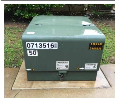
Eagle's Landing Building 13 Transformer (T18)
