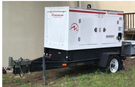
Mobile Building 1 Portable Generator (G6)
