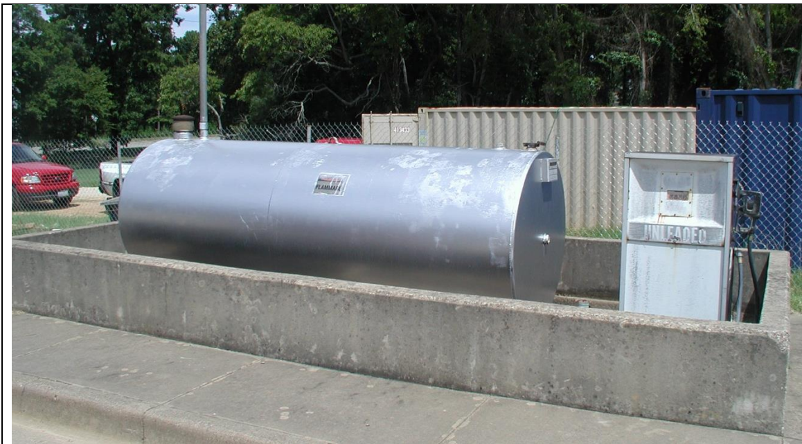
PHY Gasoline Storage Tank (AST4)
