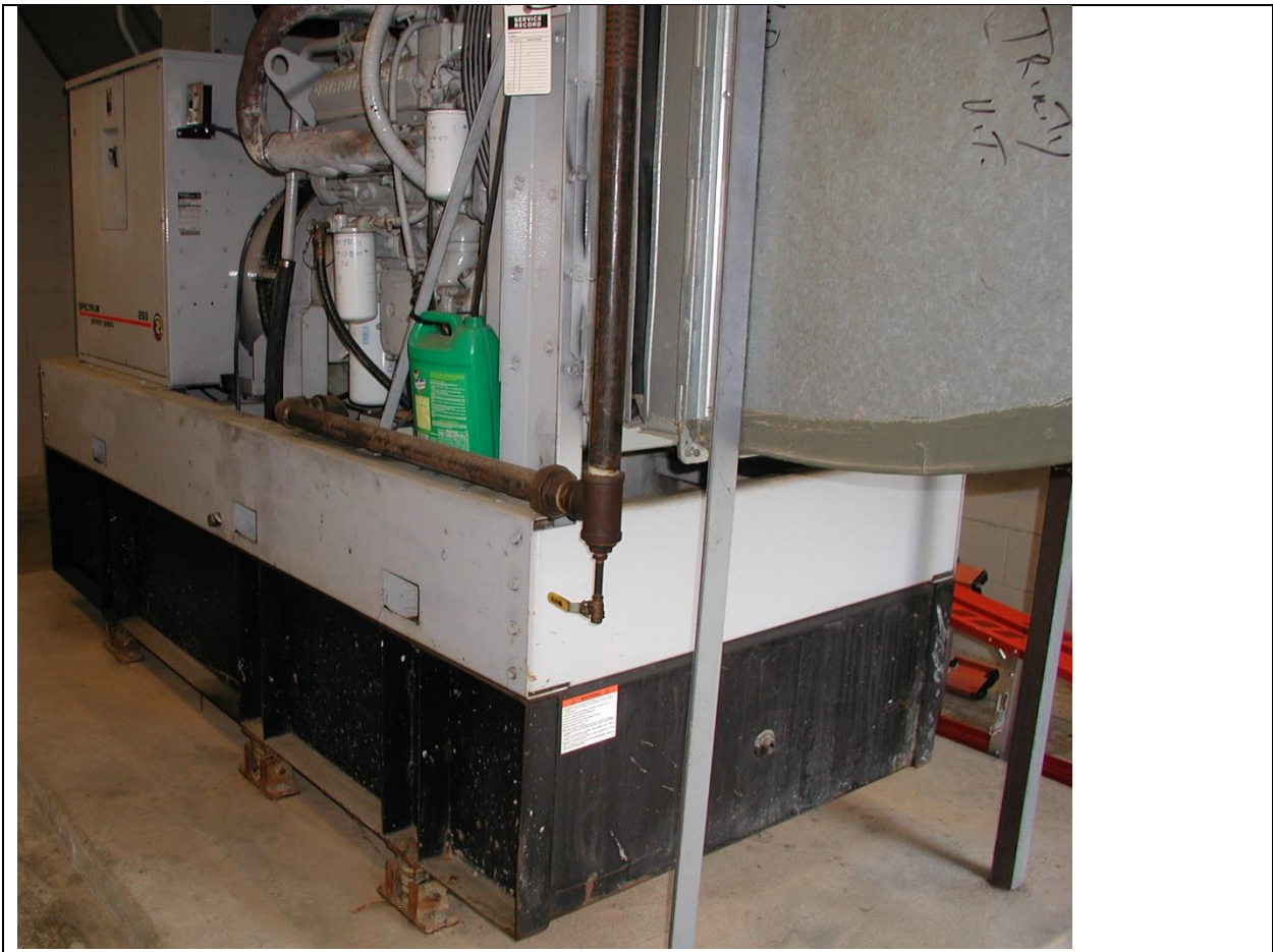
FAC Generator (G1)
