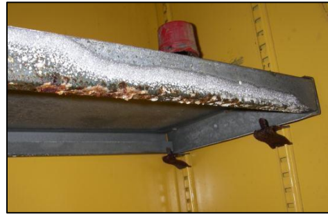
Corroded shelf supports
