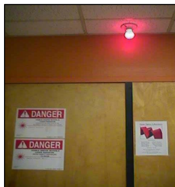
Laser warning light
