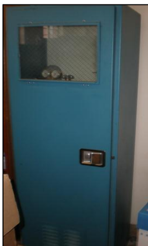
Compressed gas cylinder cabinet
