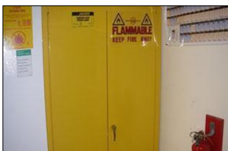
Proper storage of flammable chemicals
