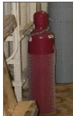
Unacceptable method of securing a cylinder
