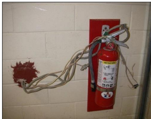
Blocked fire extinguisher
