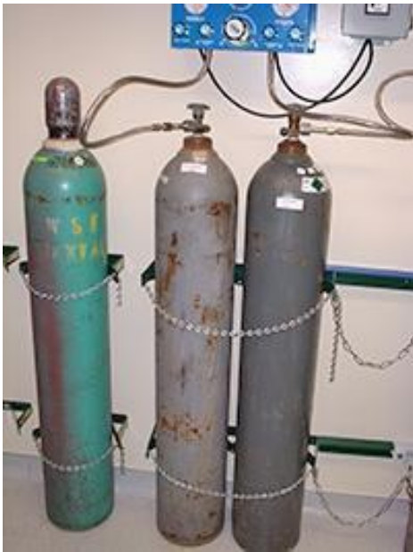
Properly restrained gas cylinders
