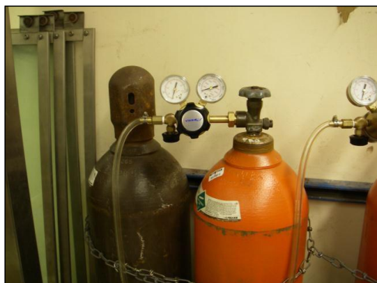
Properly attached regulator and safety cap
